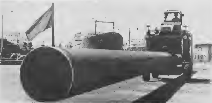
TWO VIEWS of sections of pipe being taken to the lank farm. Several times the length of the Ross carrier, the pipe in transit makes an interesting sight.
